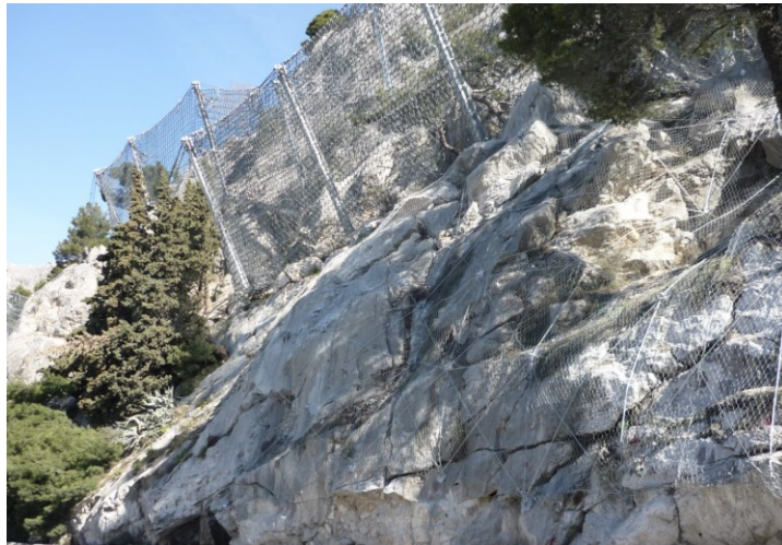
Figure 5 Protective net-protection against the rock fall (Geotech, 2024)
