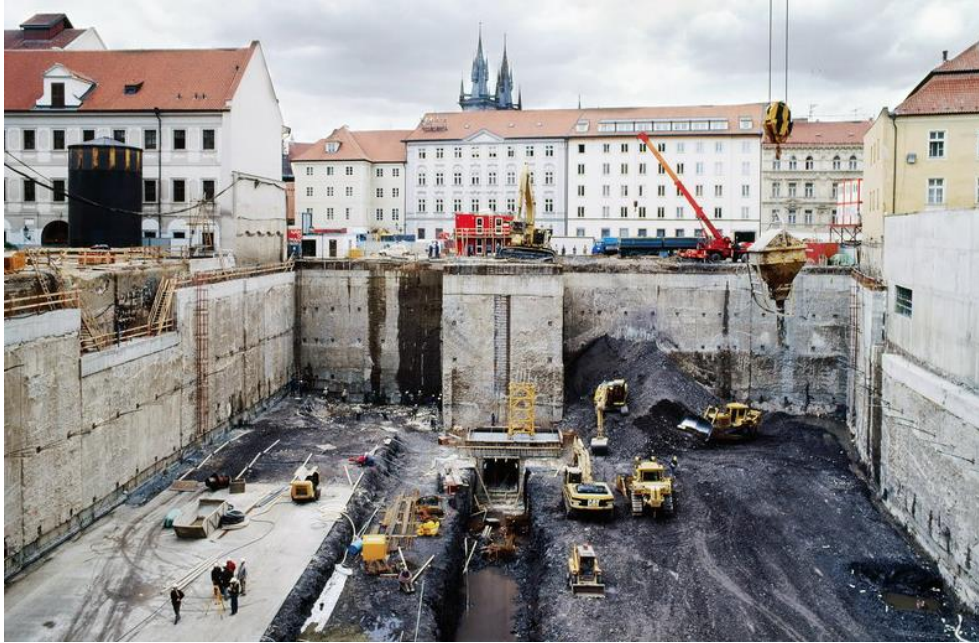
Figure 1 An example of excavation of rock material in an urban area (Zakladani, 2023)
