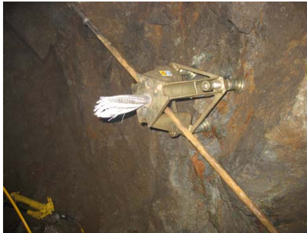
Figure 4 - Broken fiberglass rockbolt
