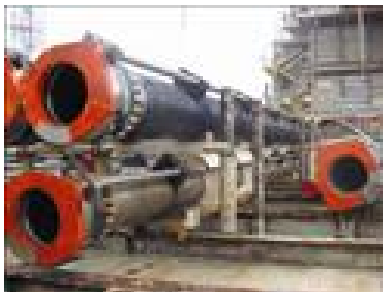
Figure 2 –Composite risers for connection of active well onto production unit "Heidrun" platform, North Sea, 2001
