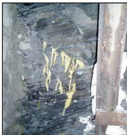
Figure 4 - Injection into fissures in the vicinity of the barrier at the coal mine in Spain
